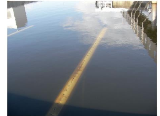
At the same time: view into the first secondary clarifier of the plant retrofitted with adapt.
